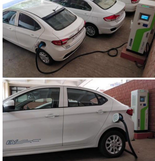
Electric Vehicle charging infrastructure at the New & Renewable Energy Department Bhopal
